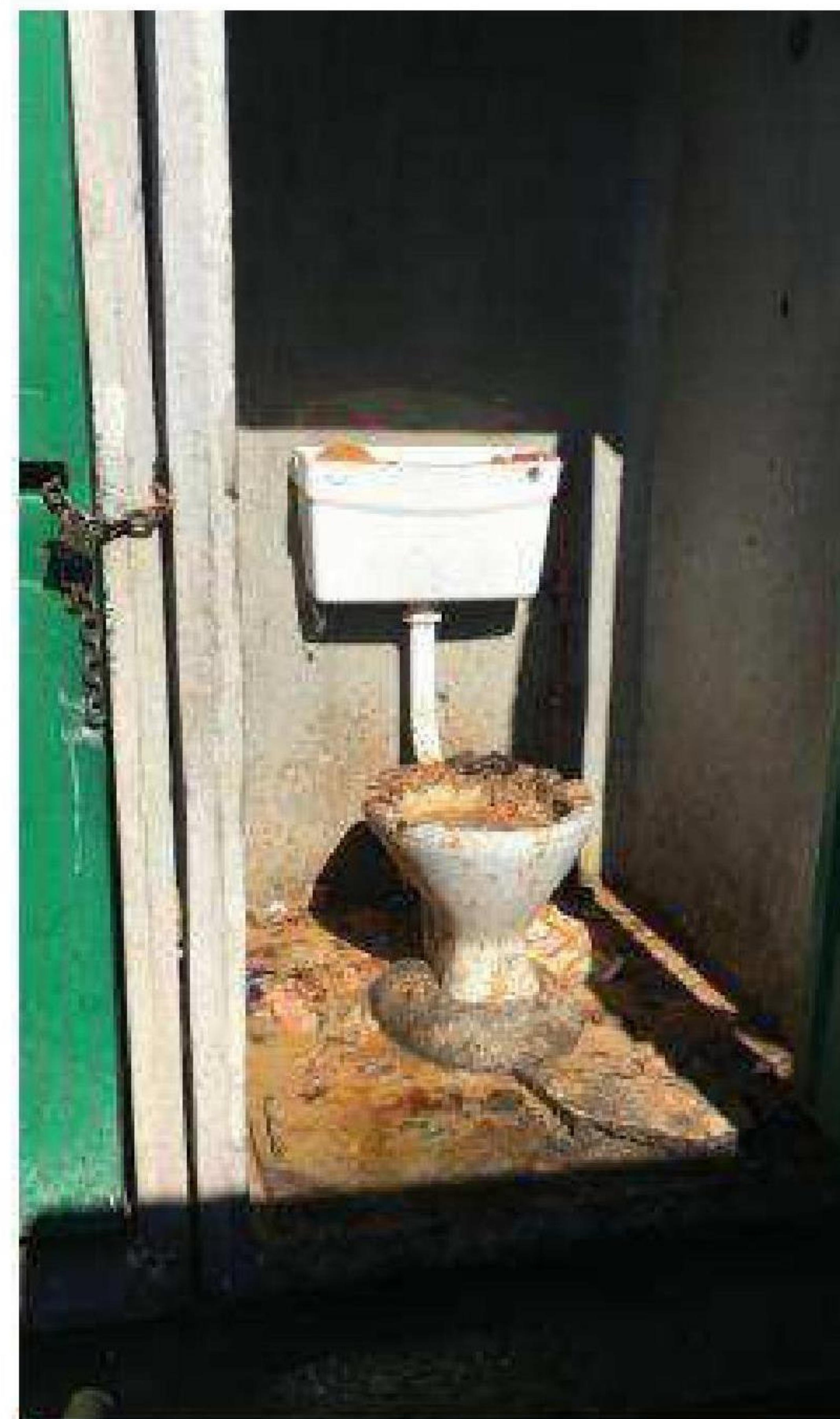
One of the blocked flush toilets catering for thousands of residents in the Ethembeni informal settlement, Dunoon. Photo. Peter Luhanga
