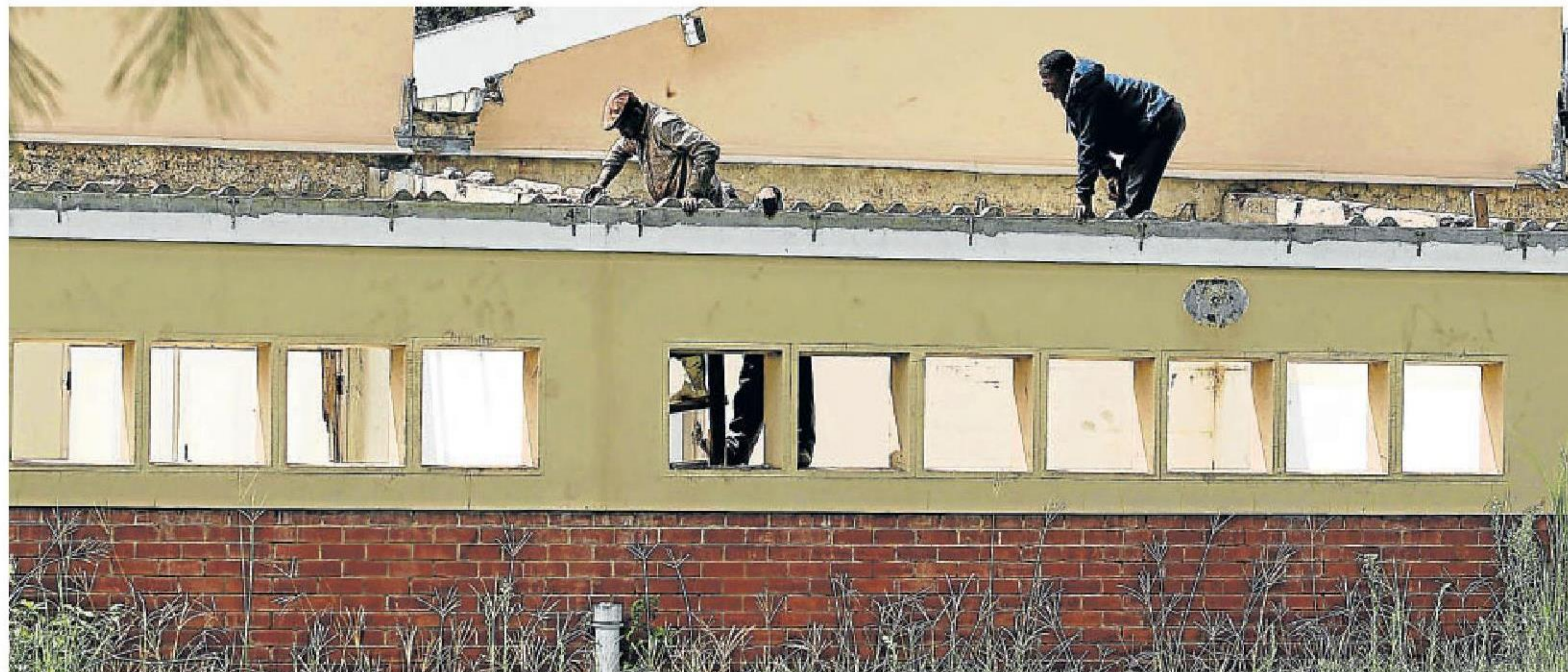
STRIPPED: The Vulindlela Technical High School in Mdantsane NU1 has been vandalised, with windows, pipes, the roof and other removable items missing. Picture: MICHAEL PINYANA
