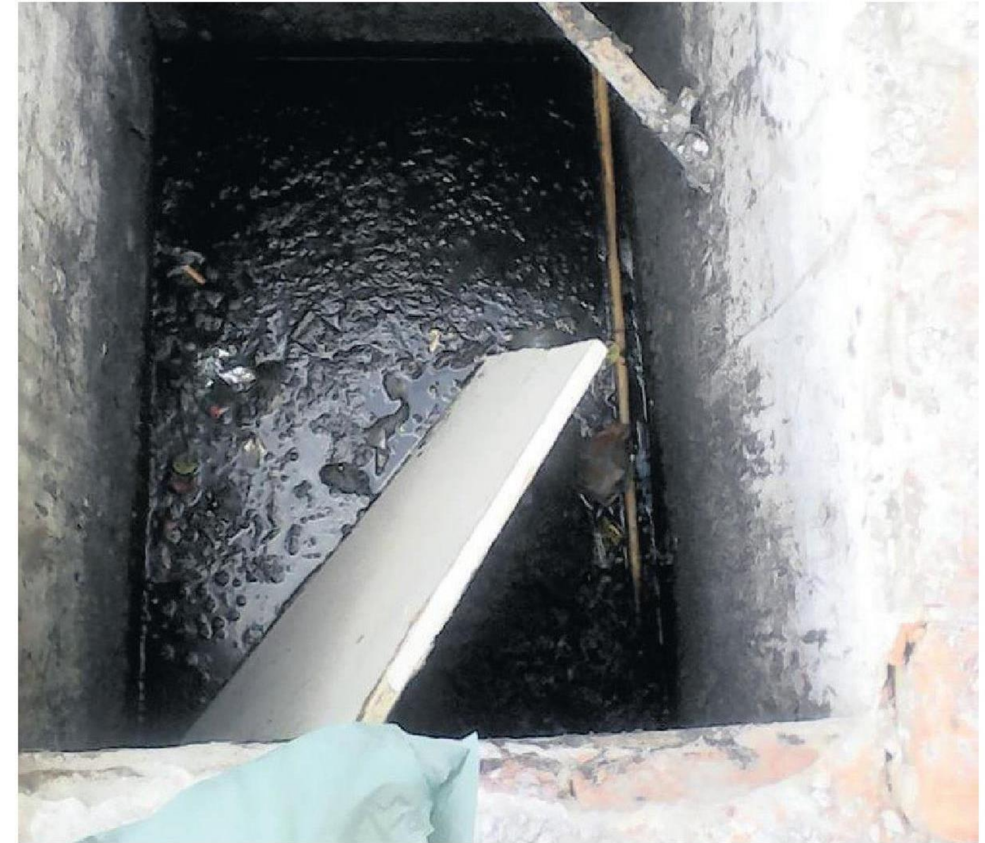
■ One of several uncovered manholes in the area.
