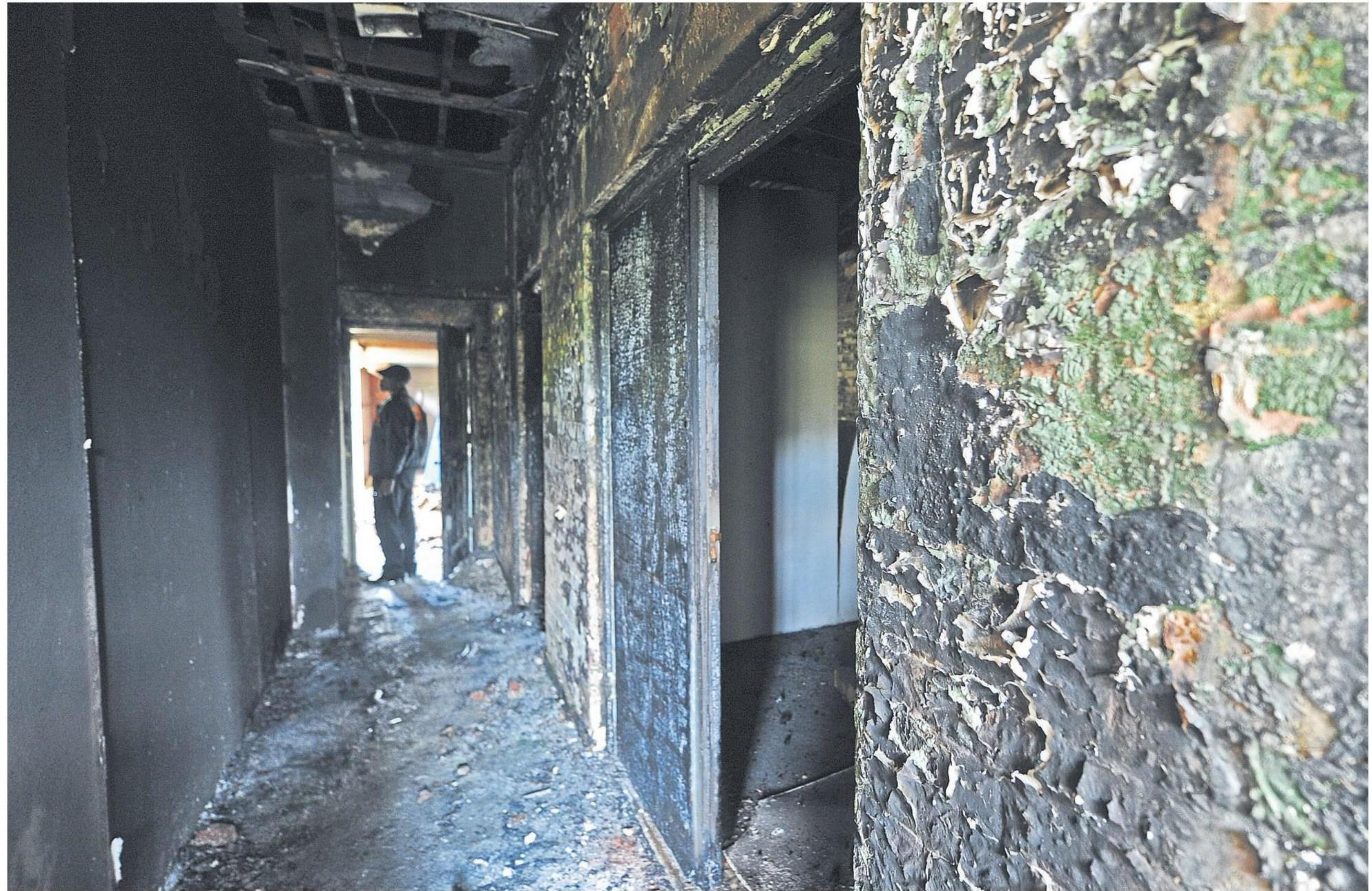
A security guard looks around the burnt out building in Oribi Village yesterday. PHOTOS: IAN CARBUTT
