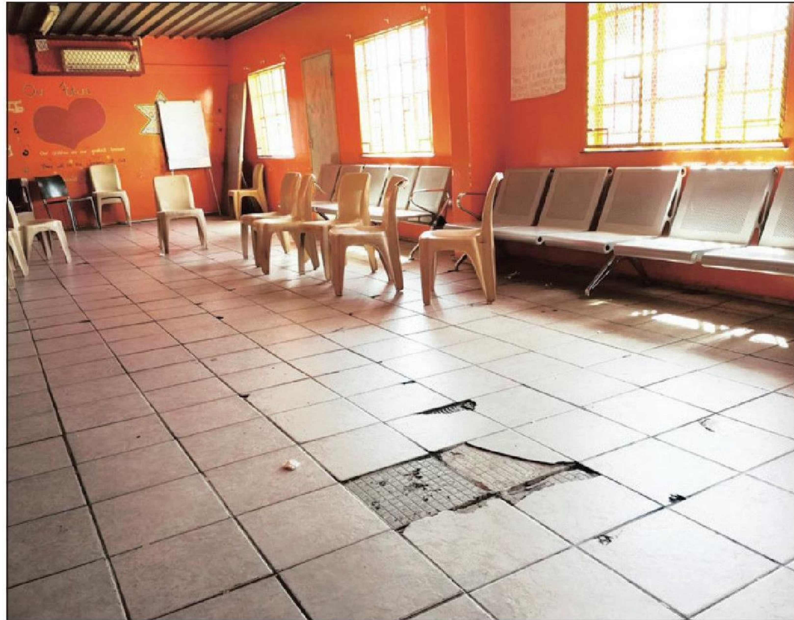
UPGRADE: The living area at the Lerato Place of Safety which forms part of the renovations which will be start soon.
