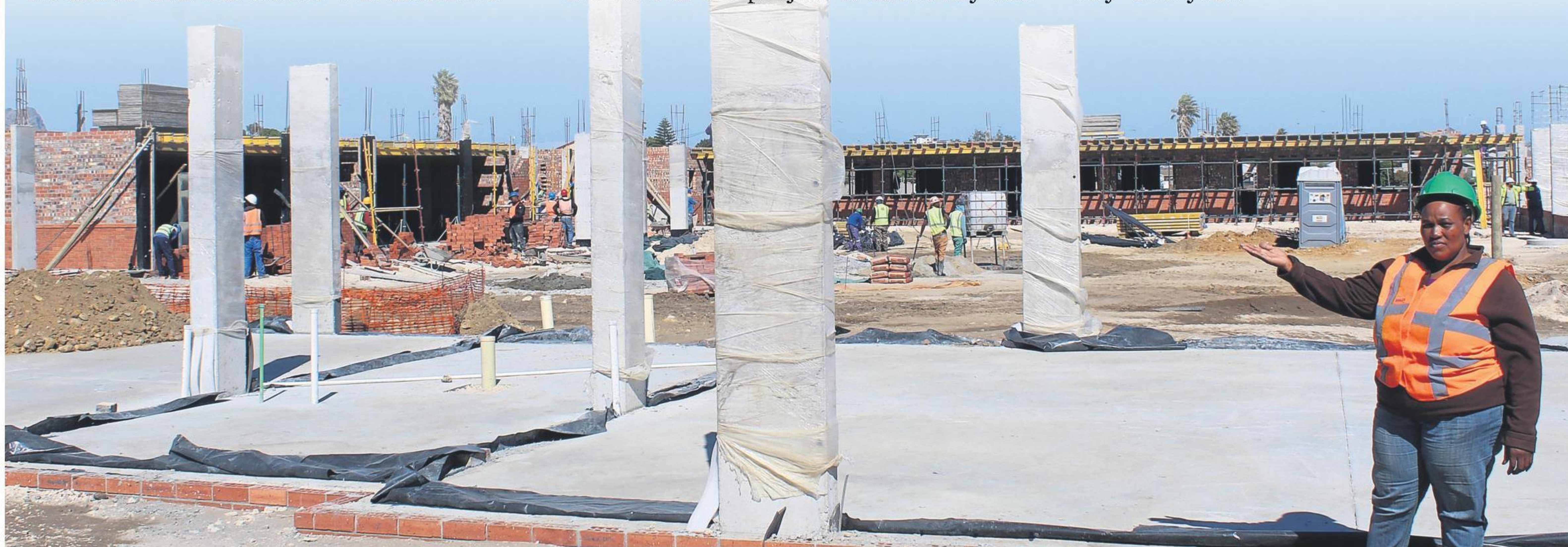
Safety officer Nomisisi Thelma Dlathu points at the construction site of the new Disa Road Primary School in Strand. PHOTO: YASEEN GAFFAR
