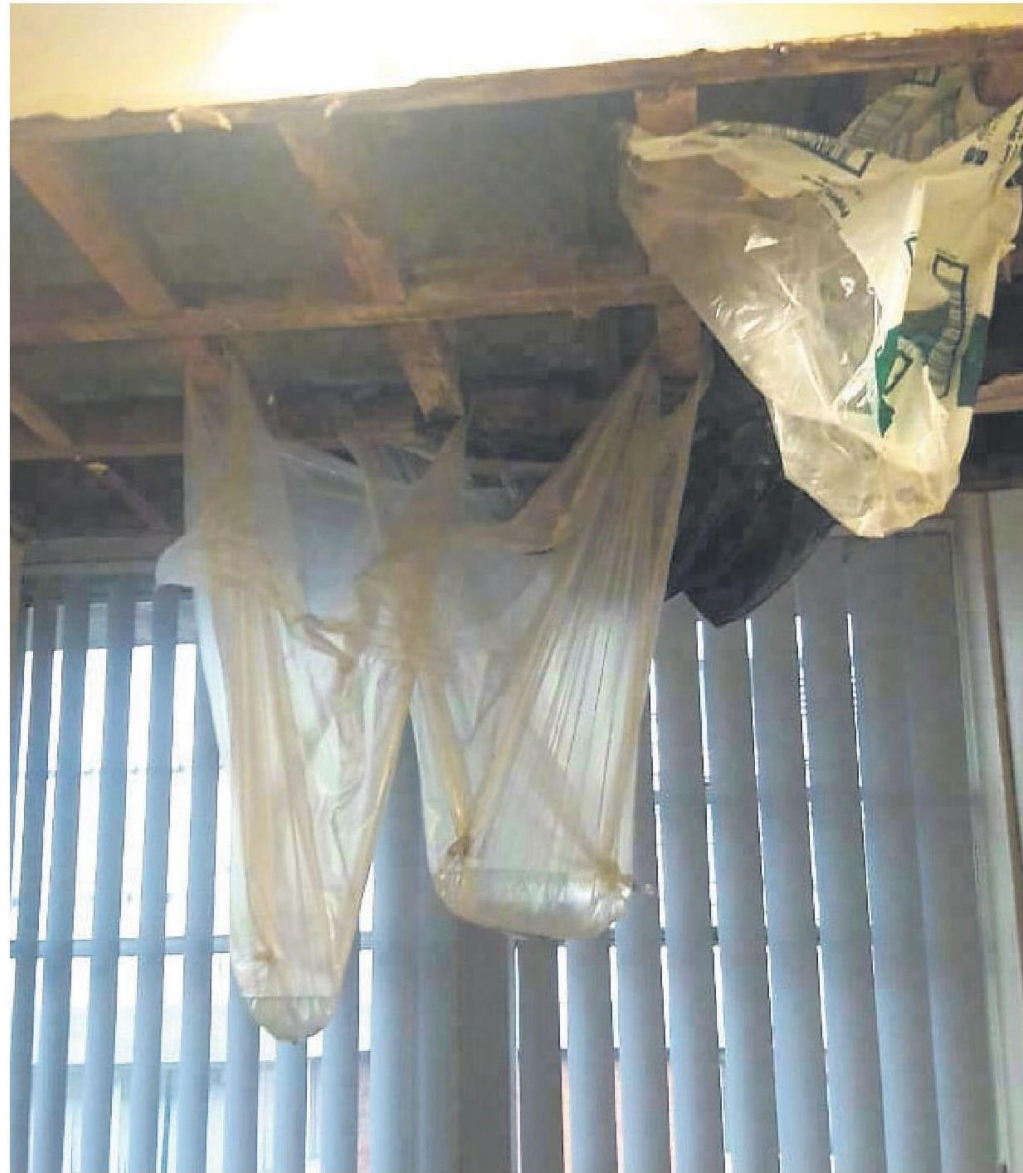
The broken roof at one of the offices at the Pietermaritzburg Deeds Office leaking onto someone's working space, with bags catching the drips.
