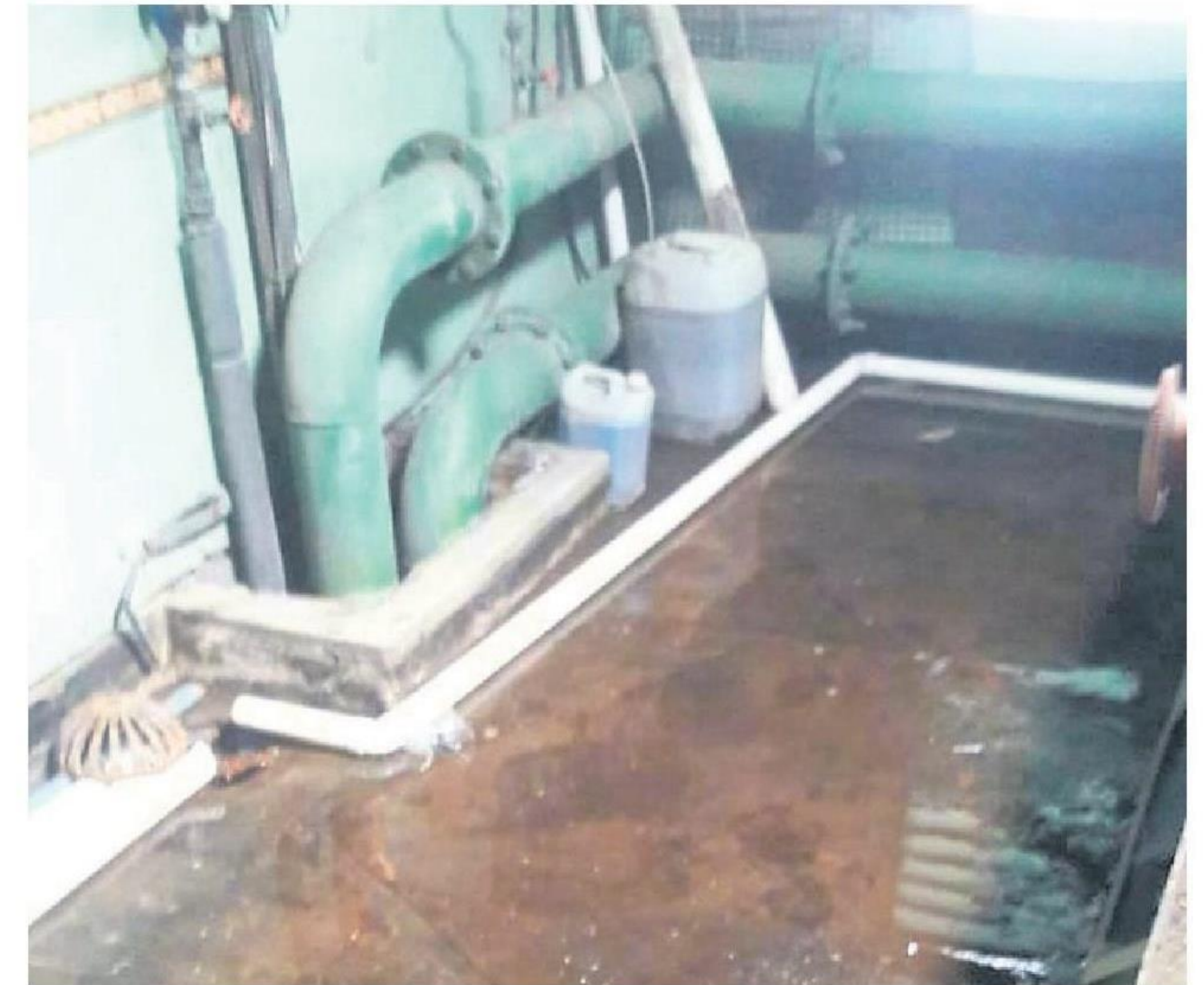
Flooding at the the Deeds Office in the city.
