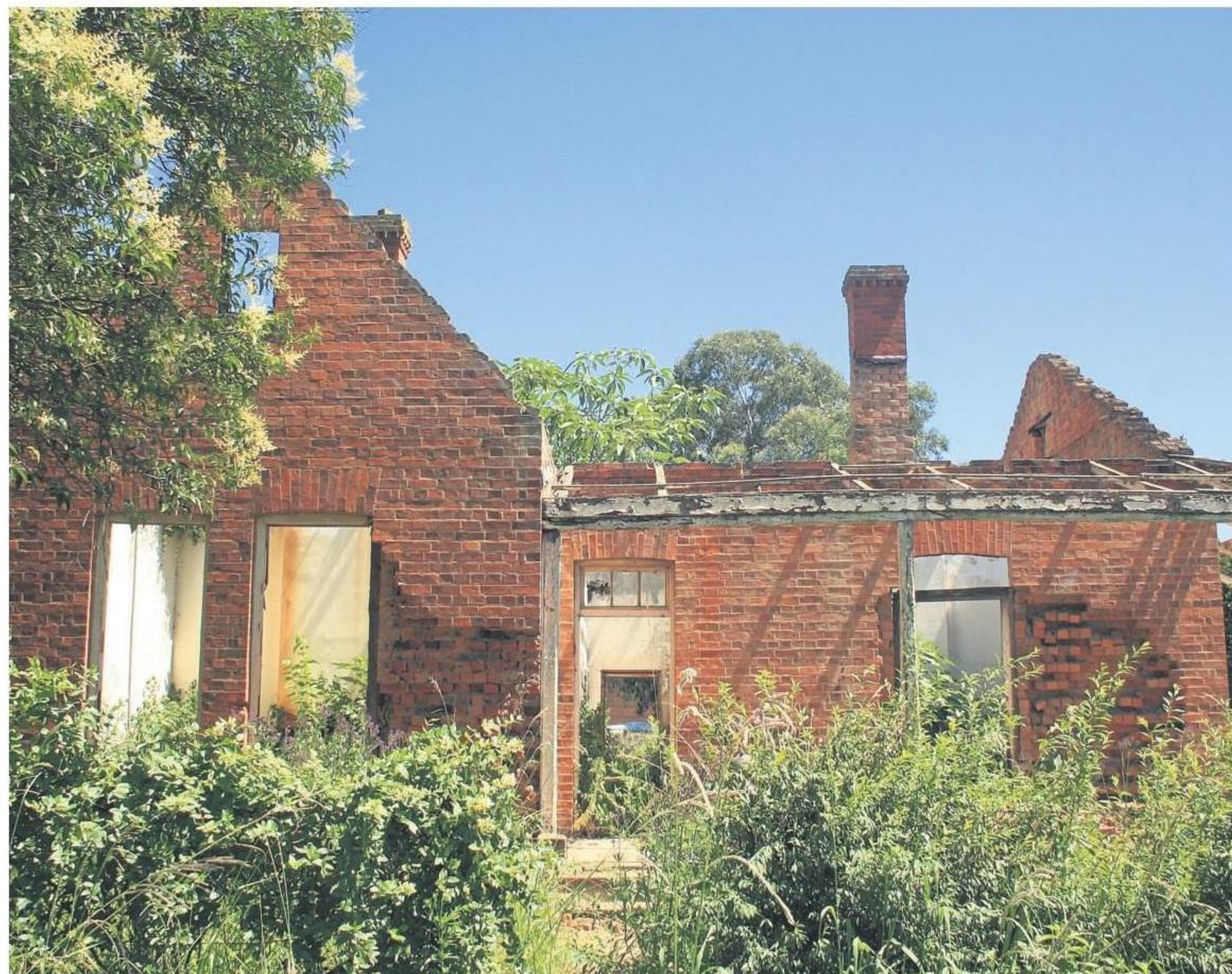
A property owned by the Department of Public Works on Morling Street in Howick has been reduced to rubble.
