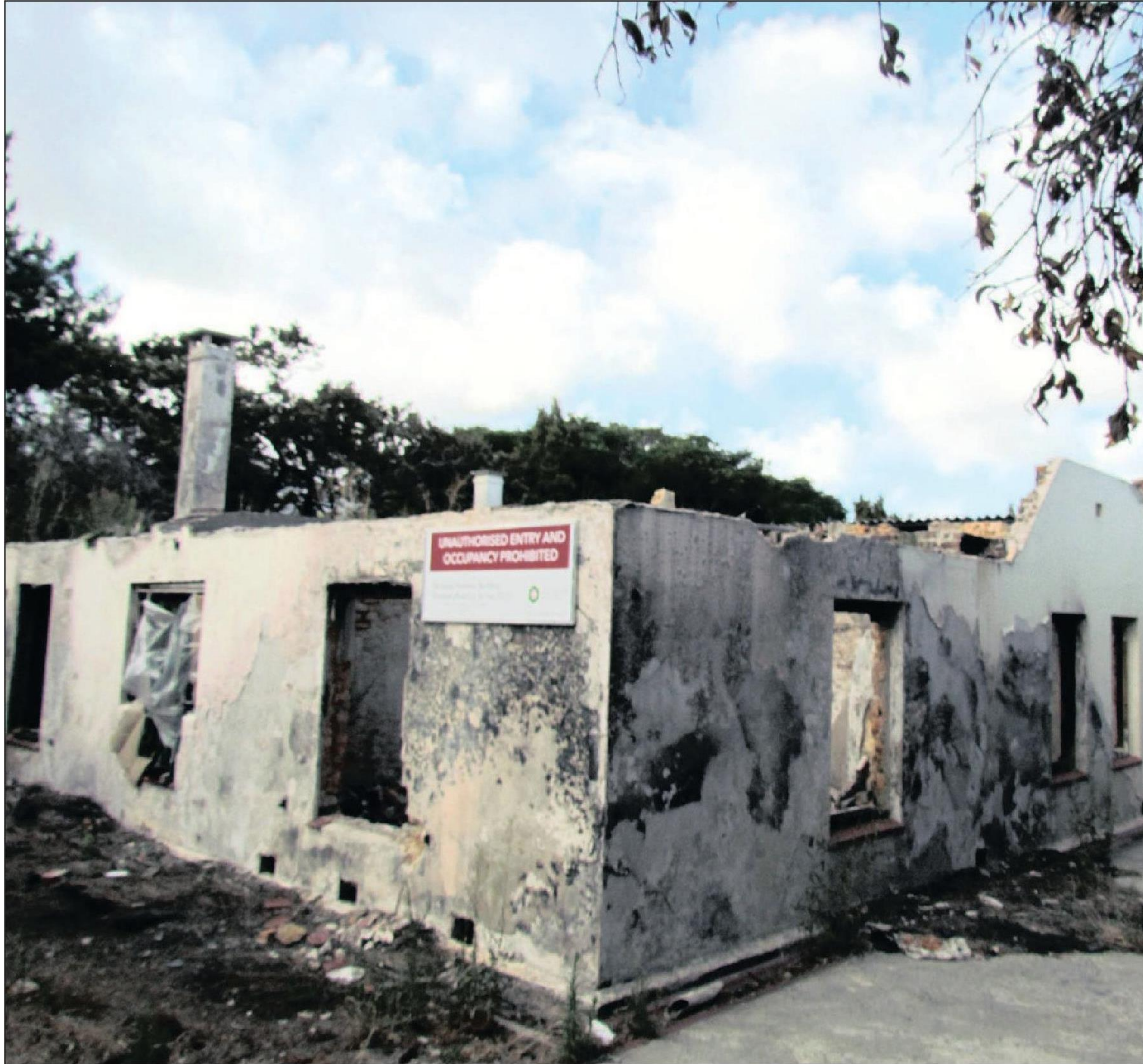
■ Ye Olde Thatch burnt beyond repair in November 2017.
