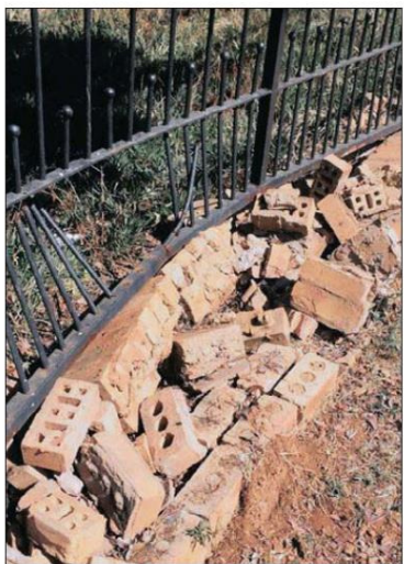
DAMAGED: Brickwork and part of the fence.
