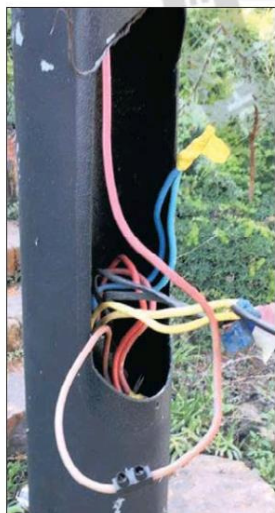
STRIPPED: No fittings for lights.
