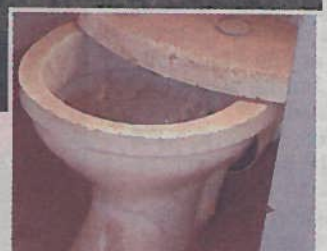
A dirty toilet in the abandoned clinic.
