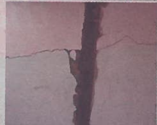
One of many cracked walls in the clinic.
