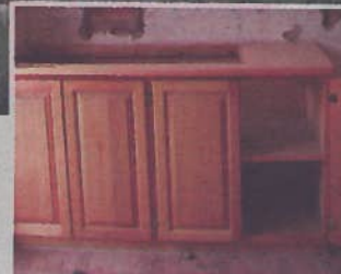
Cupboards in the building have been vandalised.
