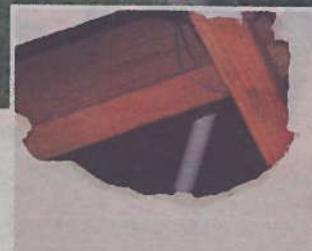
A hole in the clinic ceiling.
